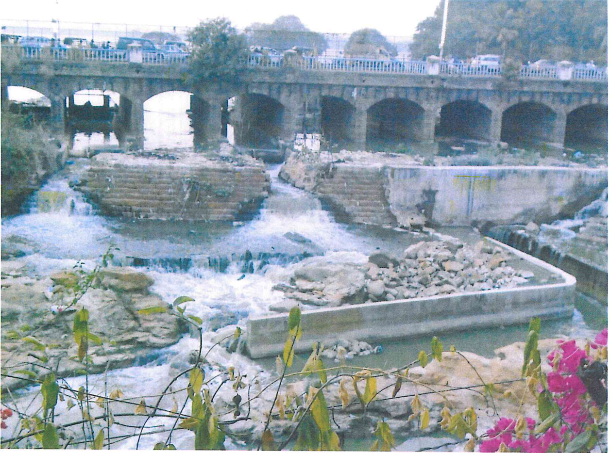
View of overflow /discharge from the Hussain Sagar Lake again confluence into the surplus channel with the stream of untreated sewage and the status of sluice gate.
