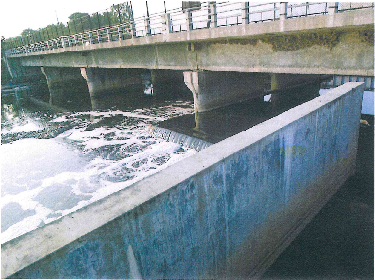
View of part of the untreated sewage directly joining in the Hussainsagar Lake from the Kukatpally Nallah.
